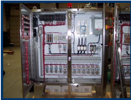
Motor Control Systems
